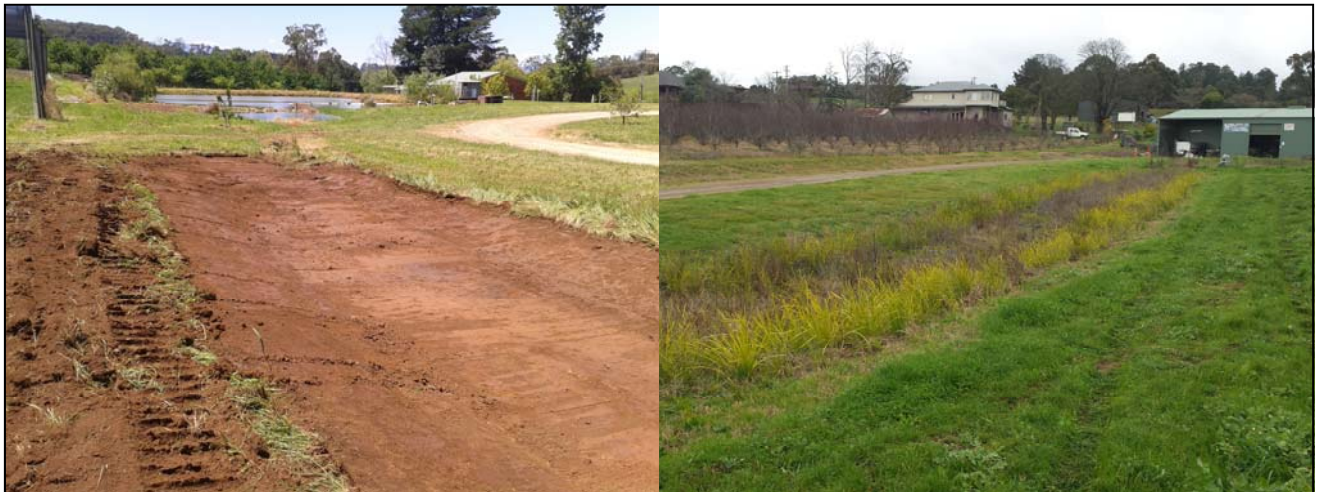
Figure 2. The constructed swale during the building phase (left), showing the trapezoid design; and after construction (right) planted with sedges and reeds.
